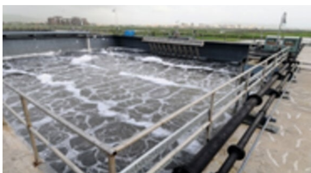
Figure 22.4 A view of sewage treatment plant
